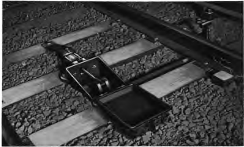
PNEUMATIC TRACK STOP, SHOWING STOP TRIGGER IN UPRIGHT POSITION
